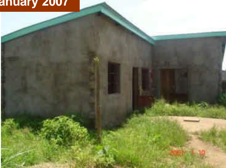
The house that Mountain Cheetah started to build for his family before running out of money
